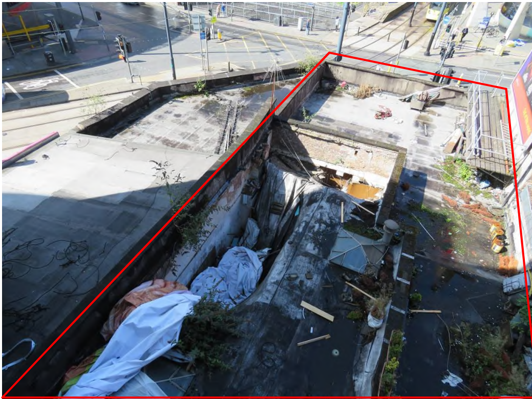
The collapsed rear of 30 - 32 Shudehill
